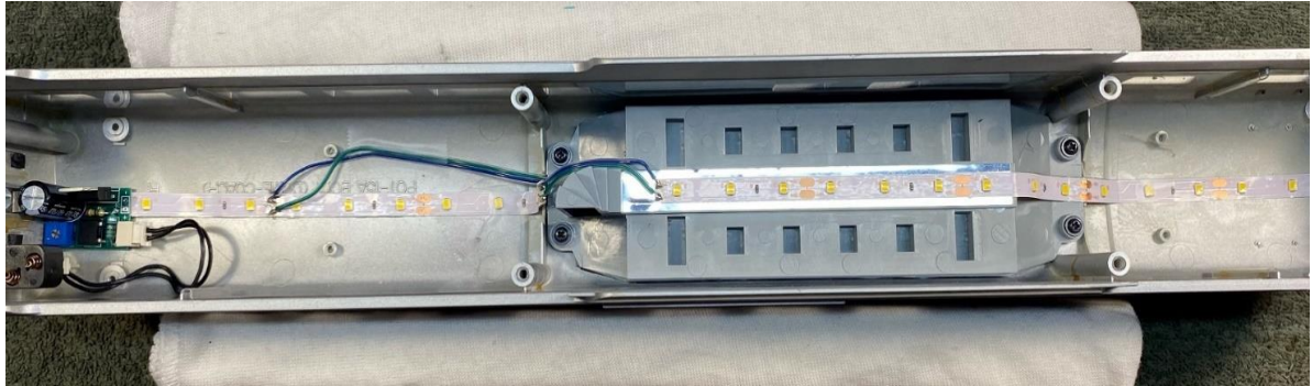
Pic 3: Typical dome car strip wiring details; both Premier and RK cars.
